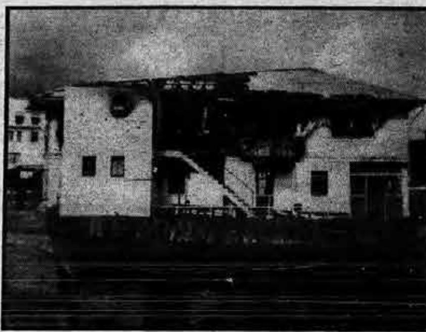
Damage done to SUP-MCS hall in Honolulu following fire is shown in photo submitted by Seafarer George E. McDonald. Fire destroyed the second deck of the building. Repairs are to be completed early this month.
