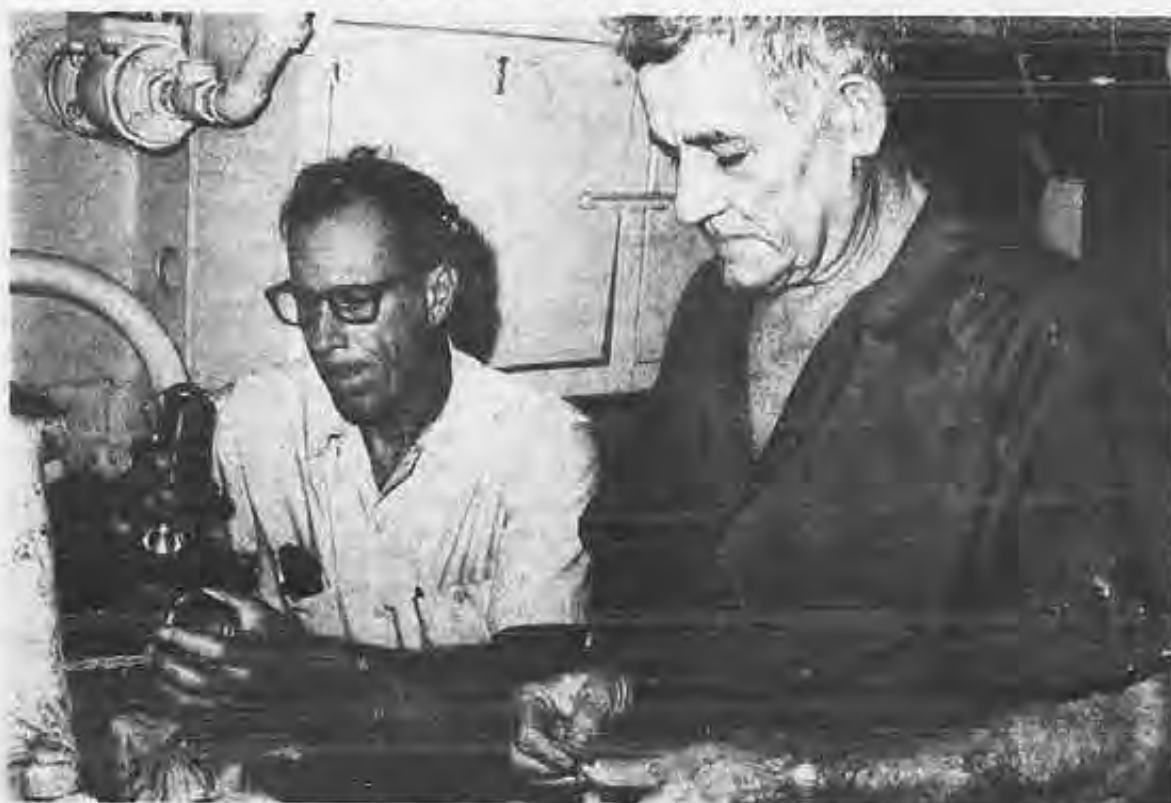
George Menge (l.), port engineer for McAllister, and Boatman John Keech, engineer, join forces to repair an air valve on the Frances K. McAllister .
