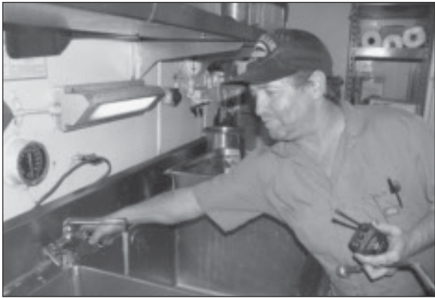
Left: Plumber Kenneth Pell checks the faucet in the galley of the Wright to ensure that water pressure is up to standard.
