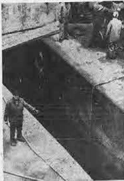
Workman points out 80-foot split in St. Lawrence Seaway back at Massena, delaying opening of '62 season.
