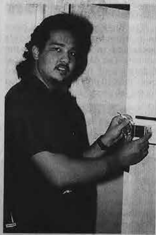
A thermostat is repaired by 2nd Reefer Engineer Bryan Chan on board Constitution.
