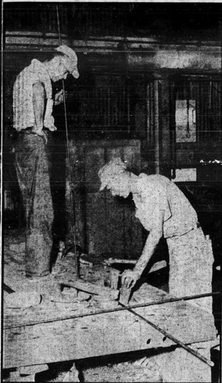
SIU-MAW members William Wilson (left) and Dan Walters bend length of pipe to specifications required in ship repair job. Many MAW members have years of Seafaring experience.
