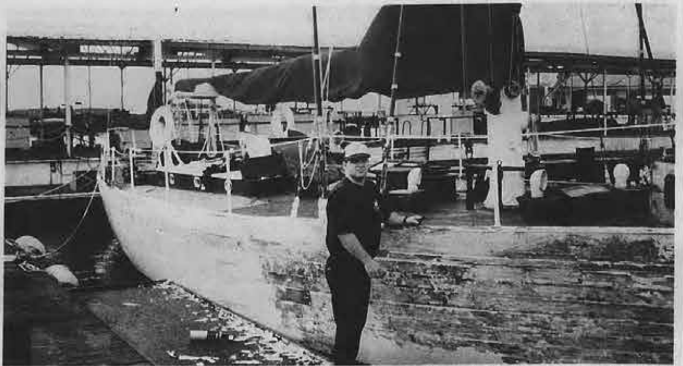
There is no shortage of work to be done aboard the Manitou to get it back into shape, as Merle Wooley finds out as he helps strip the hull to prepare it for priming and then painting.
