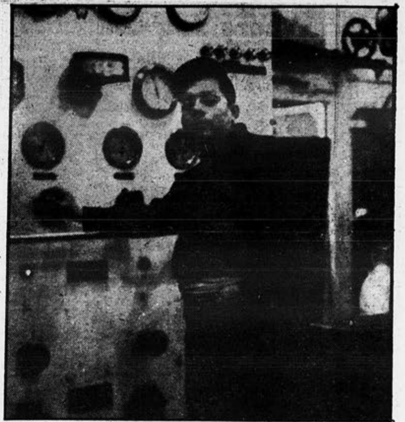
Estaurdo Cuenca, fireman, stands watch in Packer's engine room. Hagan boilers on ship are tough to handle, he says.
