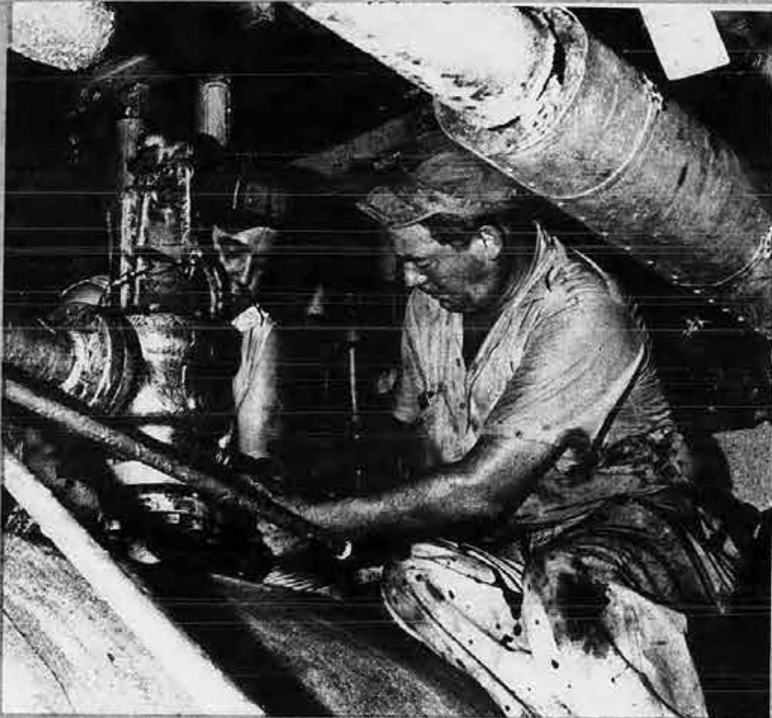
Charles Michaels, 2nd assistant engineer, at right, and Dale Chambers, oiler, make a final check on the boiler drum safety valve drain line before sailing. Michaels got his 3rd assistant's license in 1966 after training at the SIU-MEBA, District 2 Engineering School, and received his 2nd assistant's license through the school in 1968.
