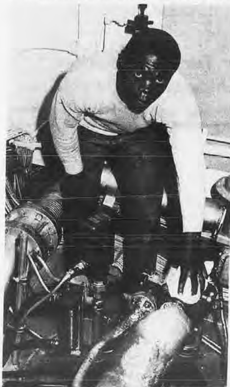
Wiper P. Sharp does some sprucing up atop one of the boilers inside the engine room's vapor hood.
