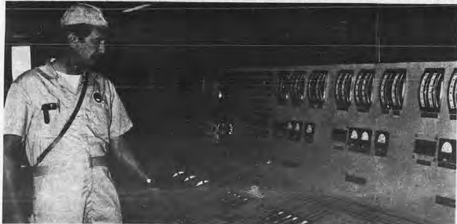
QMED Don Busby checks the readouts of Cargo Tank No. 3 from the displays on the Cargo Control Console. From here he is able to check the level of inert gases in the tank, as well as the temperature and pressure of the tank.
