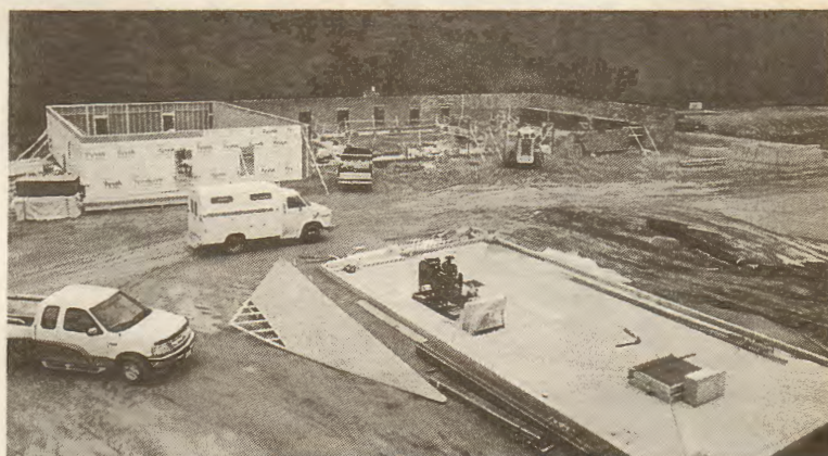
Although many areas of the country have been blitzed by severe weather this winter, Maryland has enjoyed a relatively mild season, which has aided construction of the Paul Hall Center's new fire fighting school. The top photo shows the burn building, which is seeking a name. (See sidebar to the left.) The other photo shows classroom sites and more.
