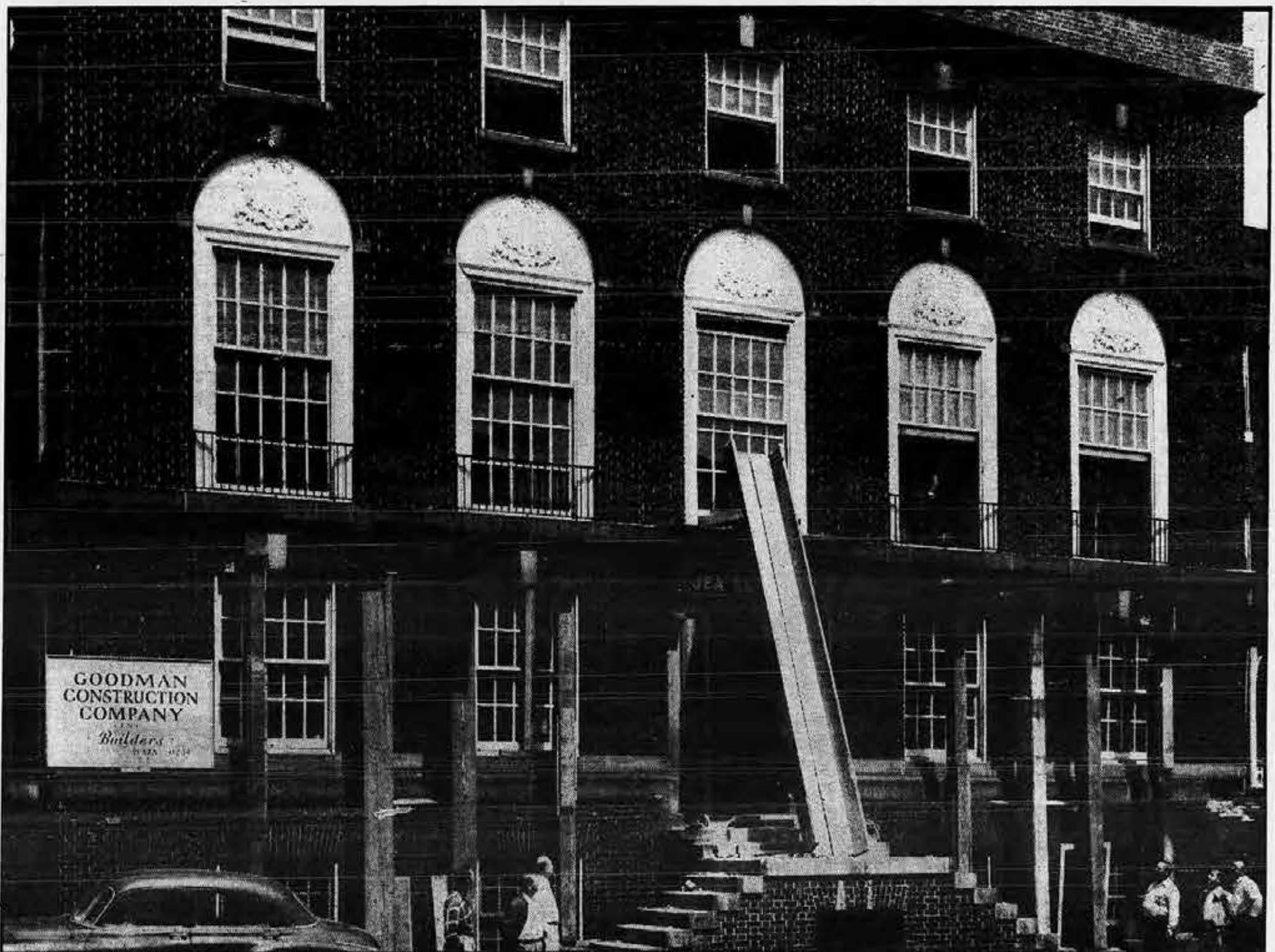
Men At Work. Under the watchful eye of Seafarer-sidewalk superintendents, work gets underway on the remodeling of the exterior and interior of the new Baltimore branch hall. Contracts have been let out for complete revamping of the building to incorporate all the facilities available in the New York headquarters. Allowing for unforeseen delays, the target date for moving into the new hall is Christmas, 1953, although it could be earlier. (Story On Page 3.)
