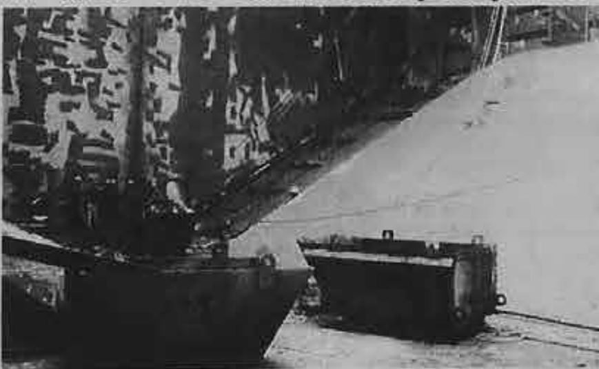
The vessel's existing cargo space was modified by removing the longitudinal bulkheads and installing upper and lower hopper plates to create a modern bulk carrier cargo hold space.
