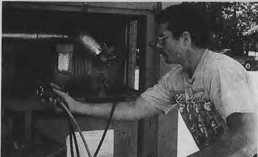
As part of the EPA Refrigeration Technician course, QMED Gary Frazier monitors the process of liquid refrigerant recovery using a site-flow indicator.
