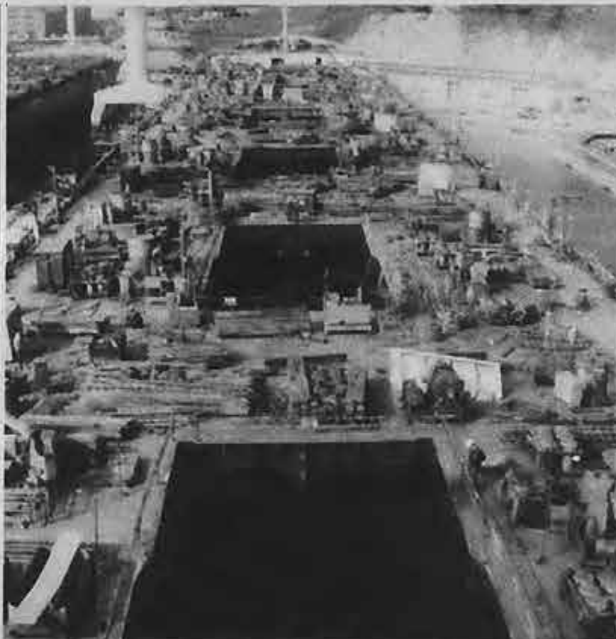
As part of the conversion process, hydraulically operated hatch covers were installed at the main deck.
