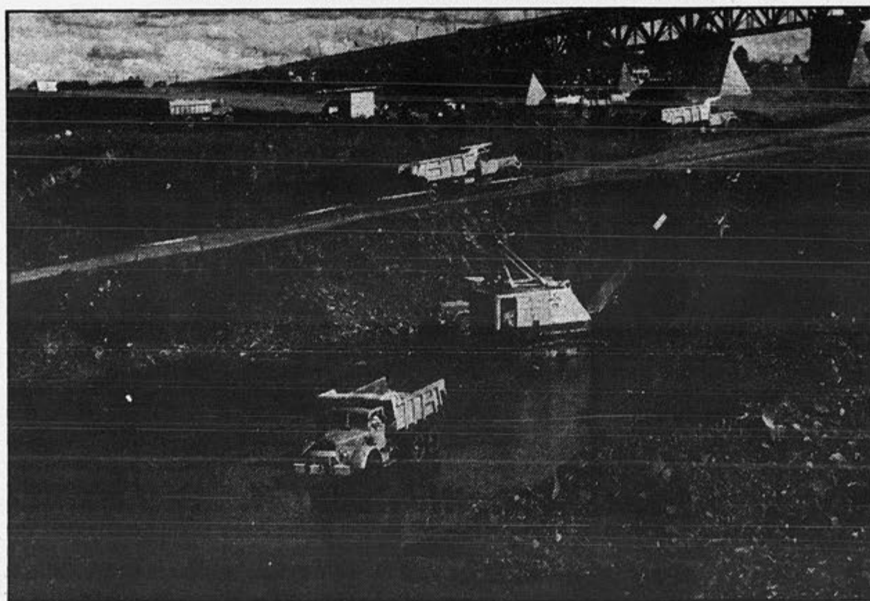
Work on the St. Lawrence Seaway is still reported proceeding on schedule, with completion now expected in time for the 1959 Lakes' shipping season. Photo taken some time ago shows excavation being done on the future entrance of the Seaway channel east of the Jacques Cartier Bridge on the south shore of the St. Lawrence River near Montreal. This phase of the project was completed almost nine months ahead of schedule. When ready, the Seaway will permit ocean-going ships to move in and out of the Lakes to the Atlantic from ports as far inland as Duluth, Minn.
