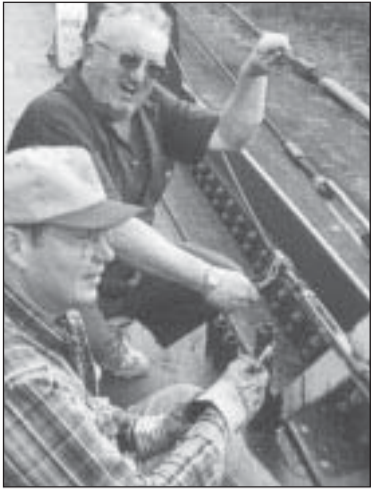
ABs Larry Curnow (top) and John Anderson work on the deck of the Joseph H. Frantz at fitout in Toledo, Ohio.
