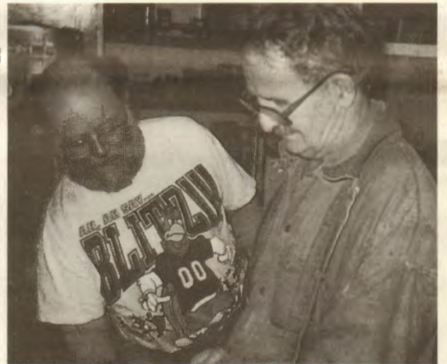
QMED Tom Curtis (left) assists Chief Electrician John Ashley in working on a breaker aboard the Cape Trinity .
