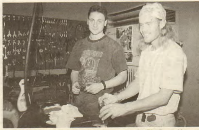
Working on a pump in the Faust's engine room are QMEDs Danny Vazquez (left) and Kevin Martin.
