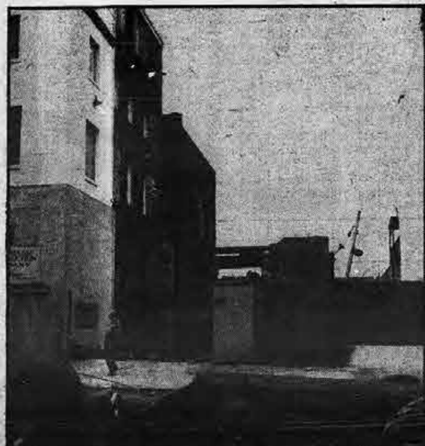
Brickwork goes up on new wing being added on the left side of the present building. It will probably be the last section of the hall to be completed.
