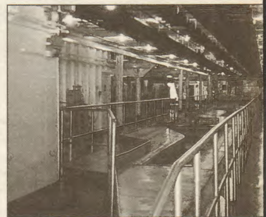
Aboard the Global Link , cable is stored in deep through machinery that helps guide it to the ocean in the area pictured directly above.
