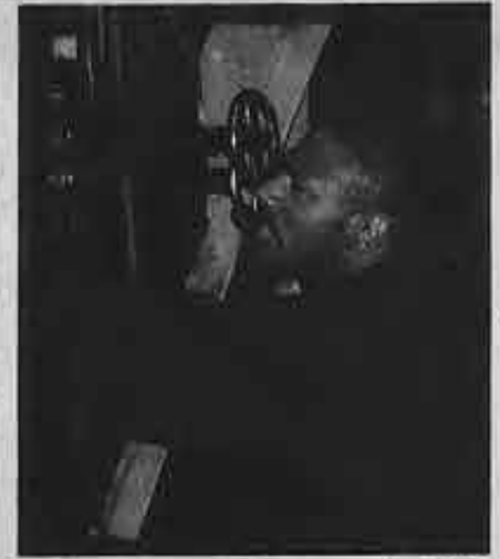
Checking the boilers on the Mississippi Queen is Douglas Kellup.
