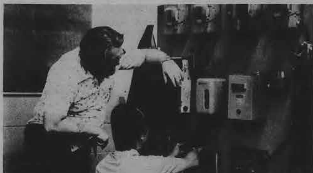
(L to R) Peter Hove, from Houston and Exequiel Liwag from Norfolk, work together wiring an electrical box.
