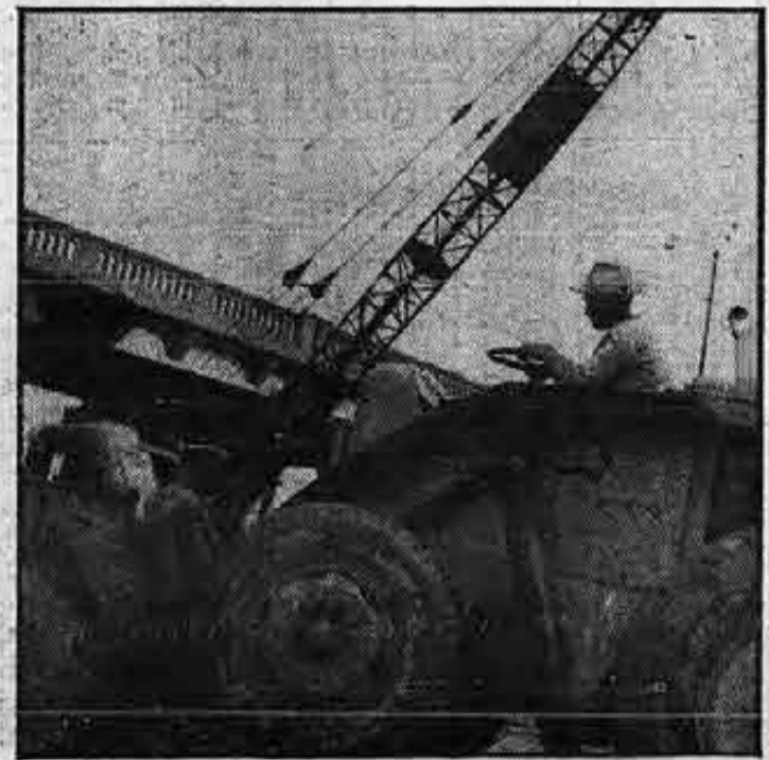
Leveling ground for new street, AFSCME member Alden Mobley jockeys truck for New Orleans' Street Maintenance Department.
