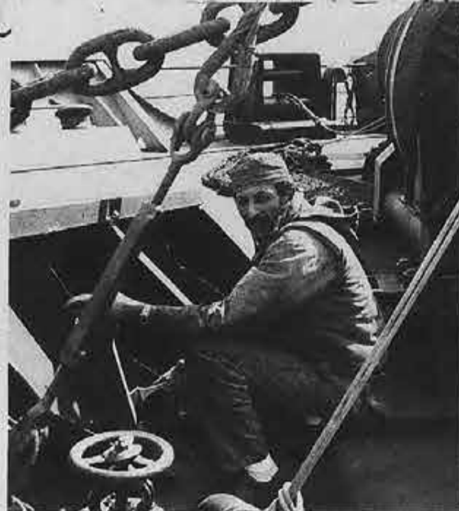
Rust-inhibiting paint is applied to parts of the deck by AB Mohamed S. Ahmed.
