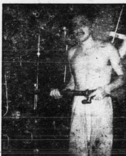
Stripped down during hot spell in fireroom, Seafarer C. Landa, fireman, is shown changing burners in a boiler on the Royal Oak. J. W. Henry, oiler, took the photo.
