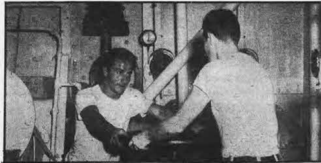
B. Gullano, Marine Firemen's Union, and 3rd assistant engineer D. McGuire, Marine Engineers Beneficial Association, get set to do some wrestling with main circulating intake.
