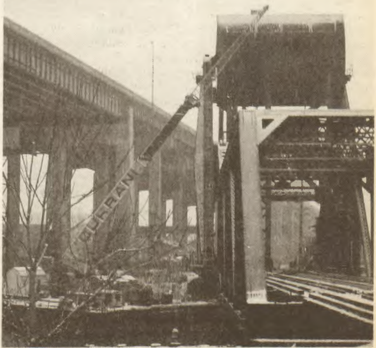
Using the crane, Seafarers prepare to lift the bridge 40 feet into the air. Massive steel columns already in place will secure the weight of the bridge before Seafarers remove the broken piece.
