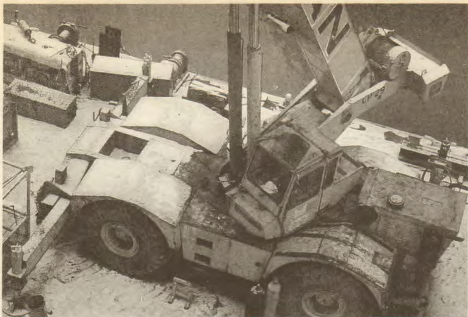
A Luedtke barge holds the large crane that lifted the River Rouge bridge so Seafarers were able to remove and replace a damaged joint.
