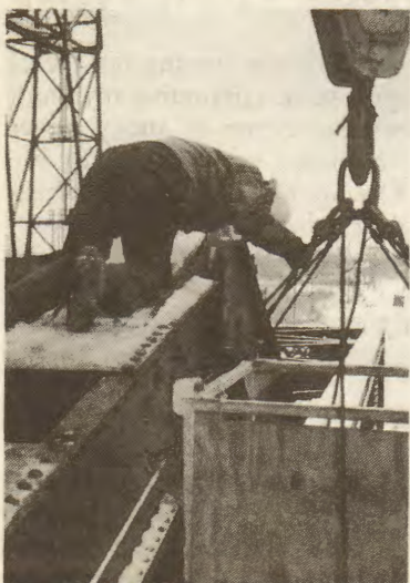
Inspecting the old bridge joint to be replaced is Dredgeman Randy Johnson.
