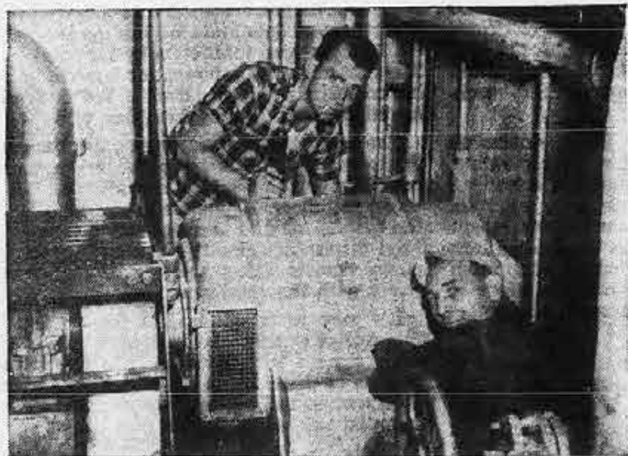
Work on generator keeps electricians George LaStrange (left) and A. E. DeLaney busy on arrival in New York.
