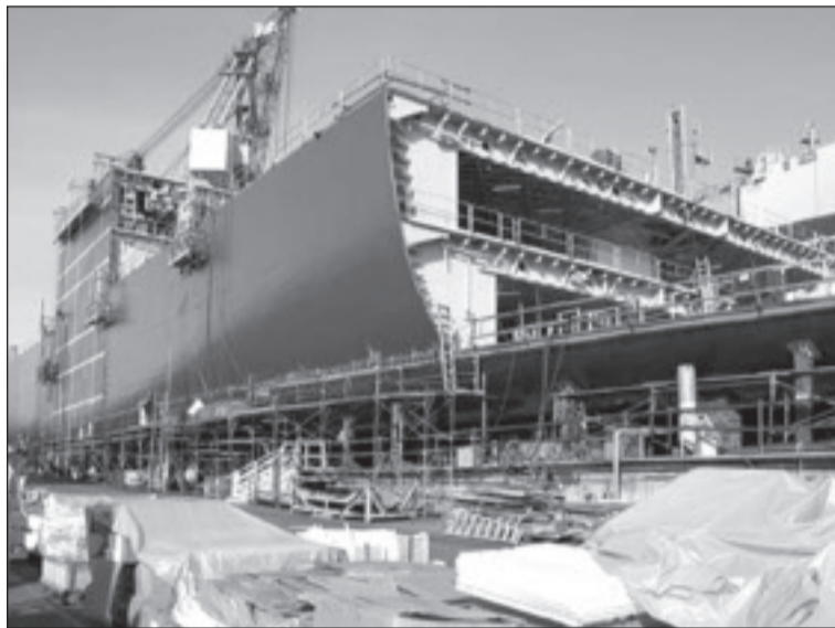
Photo courtesy General Dynamics NASSCO The fifth T-AKE ship, the USNS Robert Peary , is under construction and scheduled for delivery in 2008.
