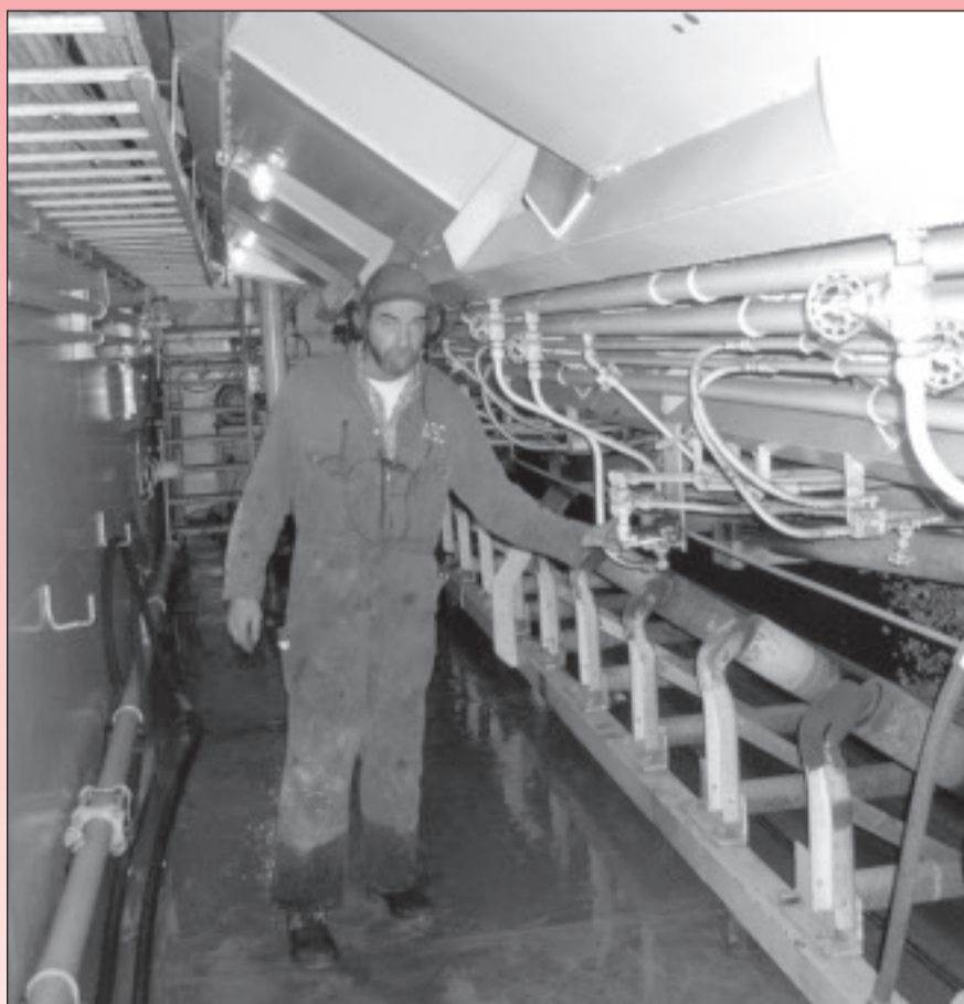
QMED/Conveyorman Jeffery Frankovich in the tunnel
