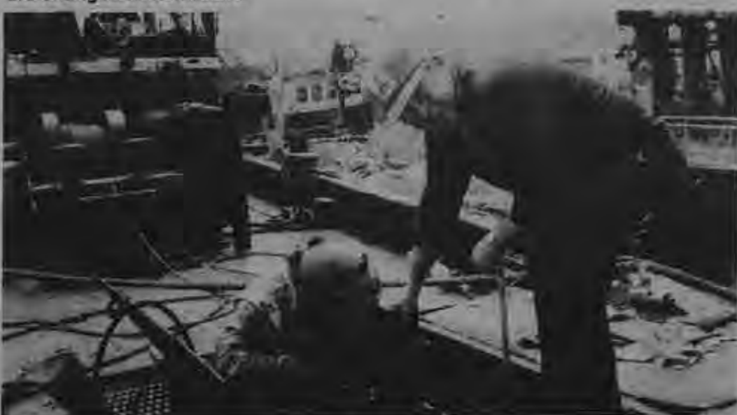
Deckhand Dan Daly (right) looks on and helps as a welder works on the tug Dugan (Dunbar & Sullivan) at the company yard in Cleveland. The very next day the tug was towing equipment to Huron, Ohio.
