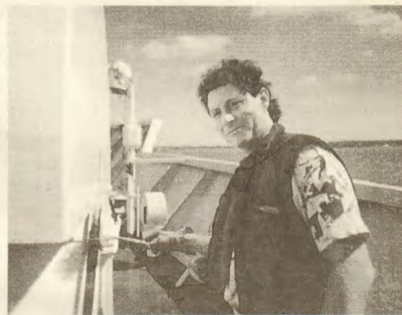
Applying a coat of paint to a vent is Cable AB Splicer/Joiner Joseph Cosentino .
