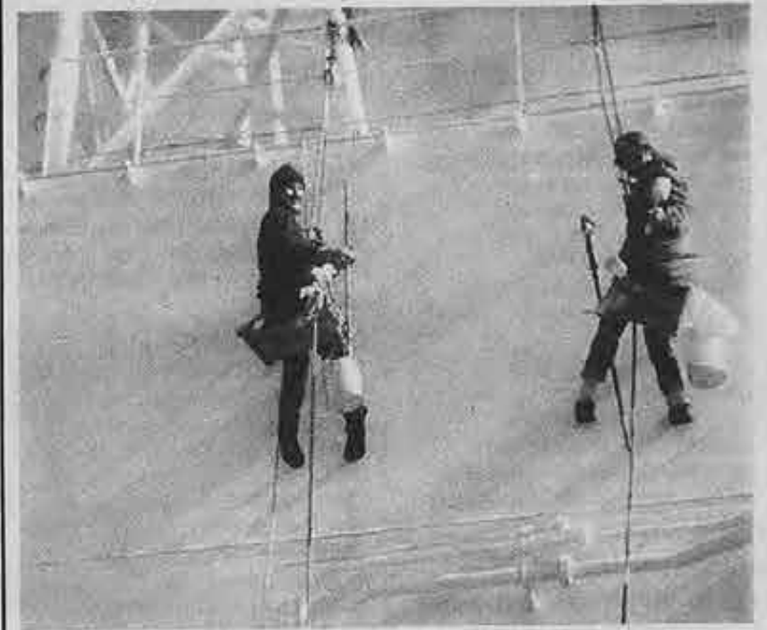
AB Mike Duggan (left) and Bosun Cesar A. Gutierrez, balanced on bosuns' chairs and with paintbrushes in hand, help keep the hull of the OMI Missouri in pristine condition.
