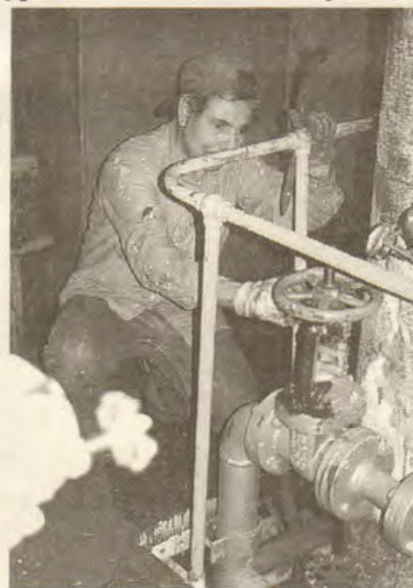
GUDE Nasser Ali adjusts a valve in the engine room aboard the Westward Venture .
