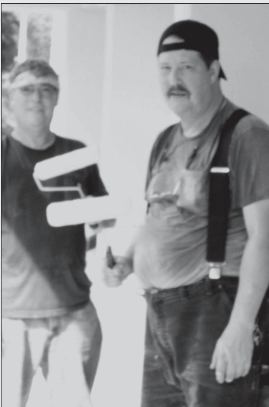
In early November, three Seafarers from the AMSEA-operated USNS 1st Lt. Jack Lummus joined other individuals in volunteering to paint the local high school in Palau during their off time. SeaBees donated the materials. SIU members pitching in included QMED Dennis Riley (left), Electrician Ursel (Buddy) Barber (right) and Storekeeper Lynne Mathison (not pictured).
