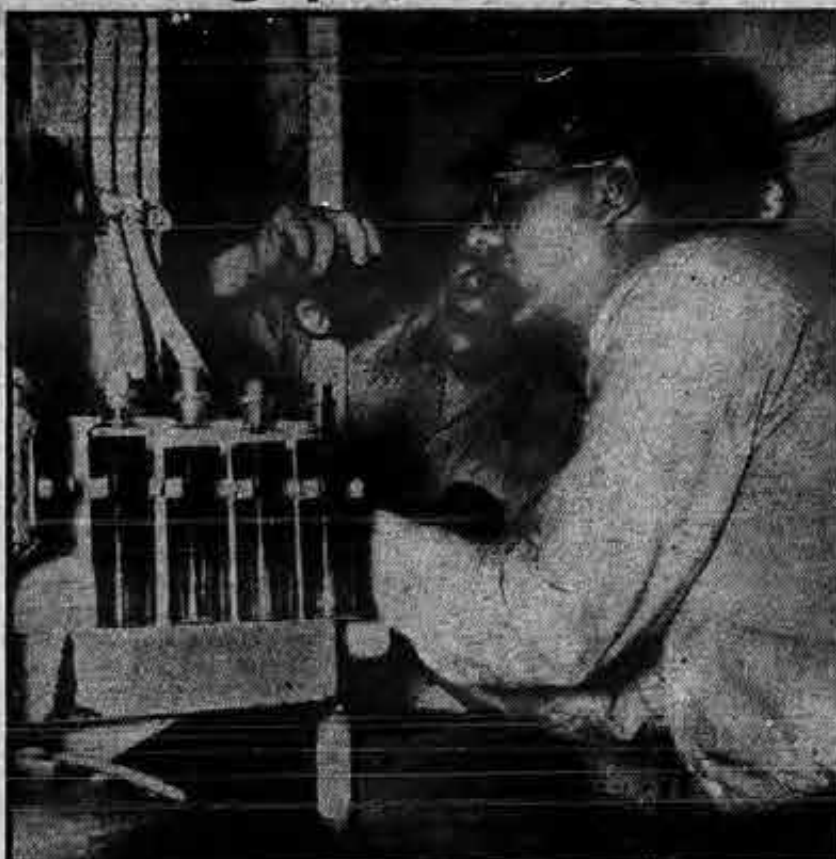
Charles Uribe (left) and D. P. Carroll, electricians on the Jefferson City Victory, are shown checking electrical cables in the ship's engine room.
