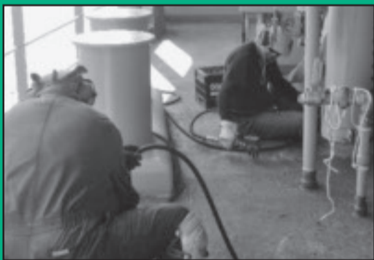
OS Gonzalo Sarra (right) uses a three-finger rust scaler while OS Gonzalo Sarra joins in chipping decks.
