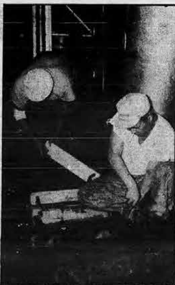
Hard at work on job of replacing broken ladder rungs are Robin Gray deck gang members Seafarers Mike Filosa, deck maintenance, and Joaquin Cortez, AB.
