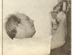
AB Jeff Gilbert removes the old sign from the front of the Fort Lauderdale building.
