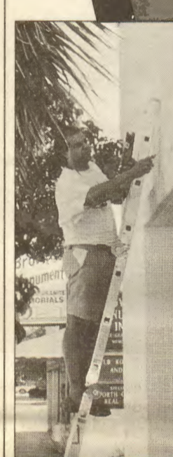
SIU Rep. Ambrose Cucinotta prepares the front of the building for the SIU logo.
