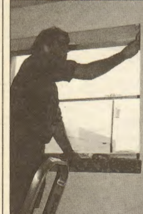
Before the opening of the new SIU office, AB Mark Ramsey repairs a window.
