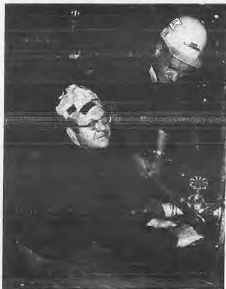
Two QMED's aboard American Steamship's Roger M. Kyes are changing the air starters in the Kyes's engine room. They are Clarence Elder (l.) and James Schutt.
