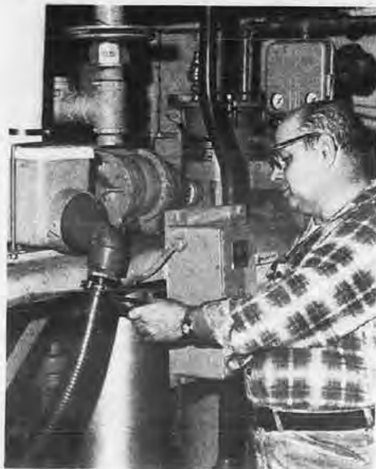
QMED Ralph Swierczynski, an SIU member since 1954, checks the Nicolet's newly installed sewage treatment equipment that's designed to cut down pollution on the Lakes.
