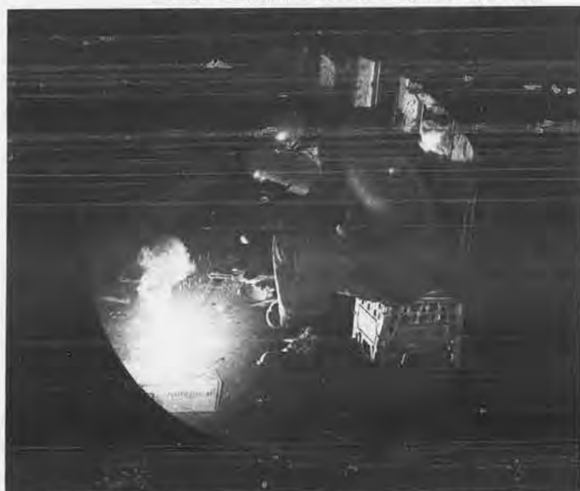
Tom Fox, an assistant conveyorman, does some welding repairs on the Cornelius .
