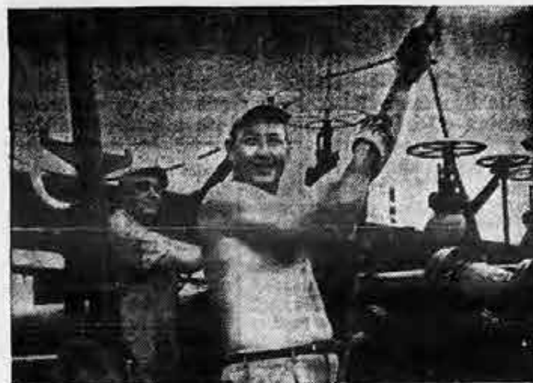
Lacey R. McAdams heaves away to raise fuel line into position for pumping operation.
