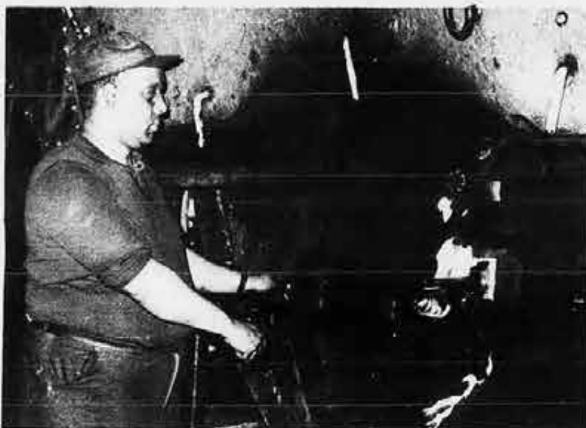
David Payne fires up one of the four boilers as the carferry prepares to get underway. An old-timer even among the other old-timers, Payne has been firing on the vessel since he first went aboard 27 years ago. He has been the SIU engine department delegate for the past 26 years.
