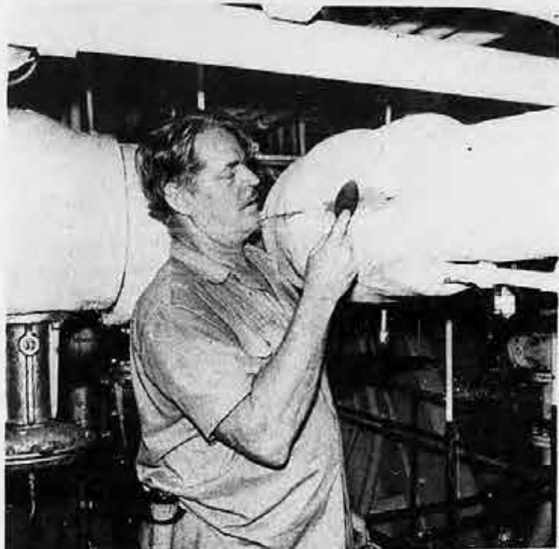
James "Rusty" Gallier, oiler, is seen here lagging insulation on a steam pipe after the ship arrived in port from St. Croix.
