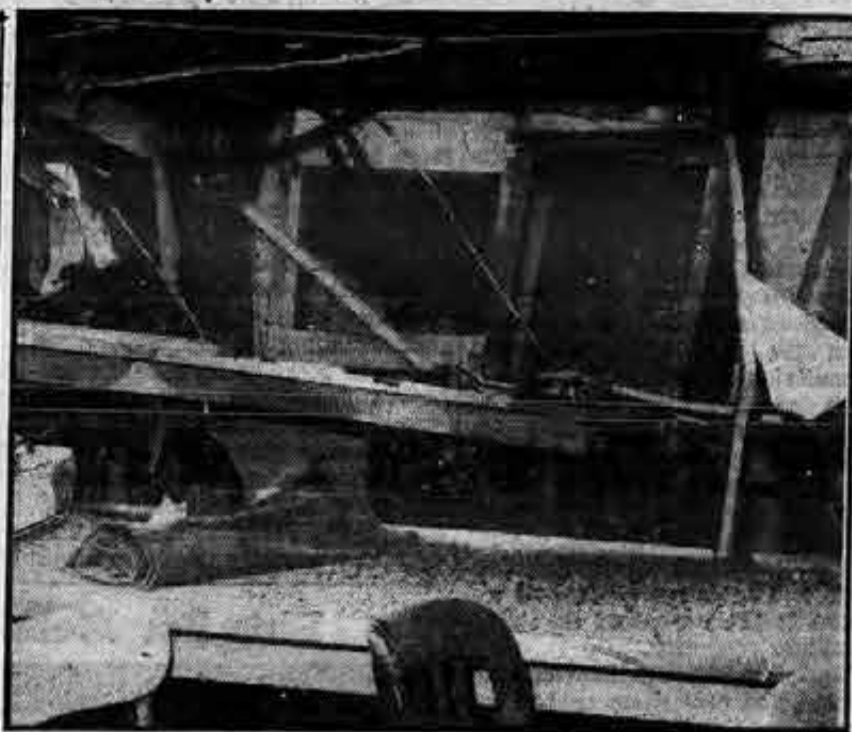
Wreckage in Valchem messroom testifies to force of impact when Santa Rosa came poling through the tanker's after house. Rosa penetrated two-thirds the way through the tanker.
