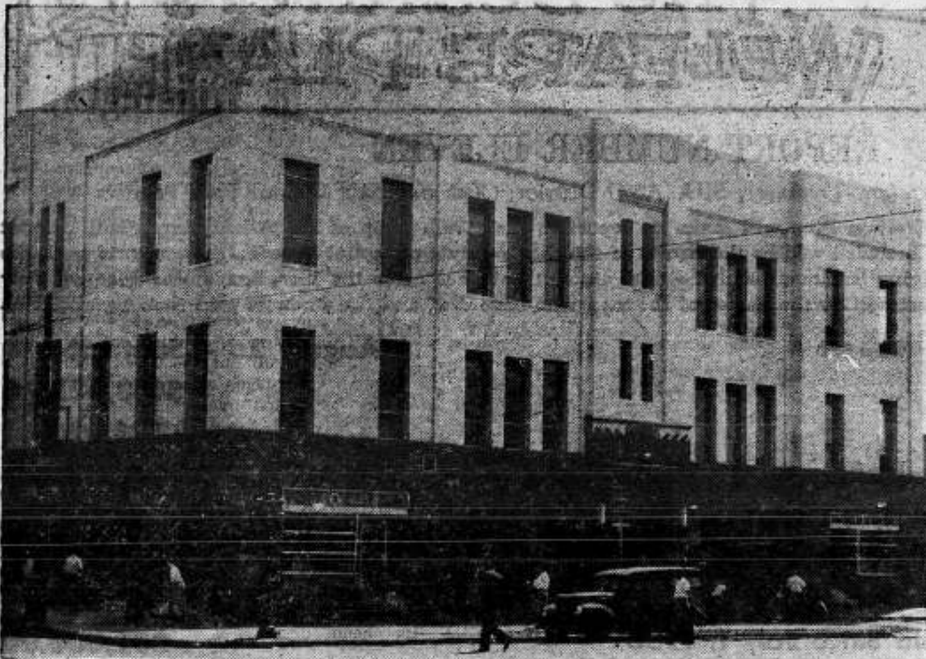
With the scaffolding removed and the iron fence torn down, the new face of the SIU's soon-to-be-occupied new Headquarters faces the sun. Inside, finishing work continues in some departments, while in others members of the Union's Headquarters staff are busy installing records and files already transferred from the New York offices.
