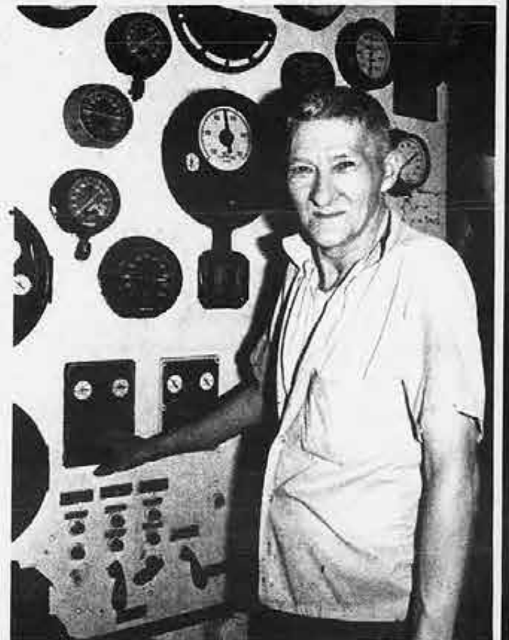
Fireman C. White checks the controls in the engine room prior to sailing again.
