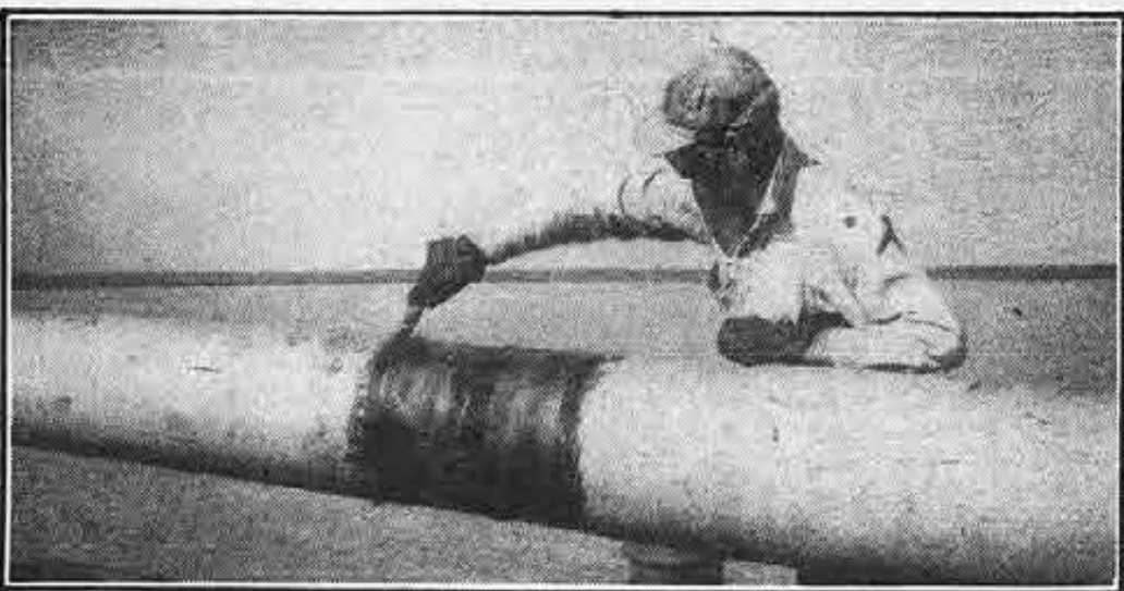
Union construction worker "primes a joint" to help seal sections of pipe used in laying gas transmission line.
