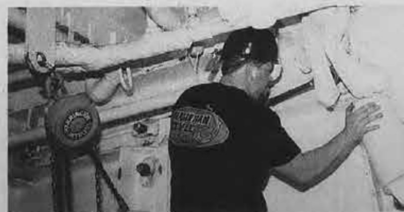
Intently loosening a large bolt on the side port is OS John "Spanky" Dunavant.
