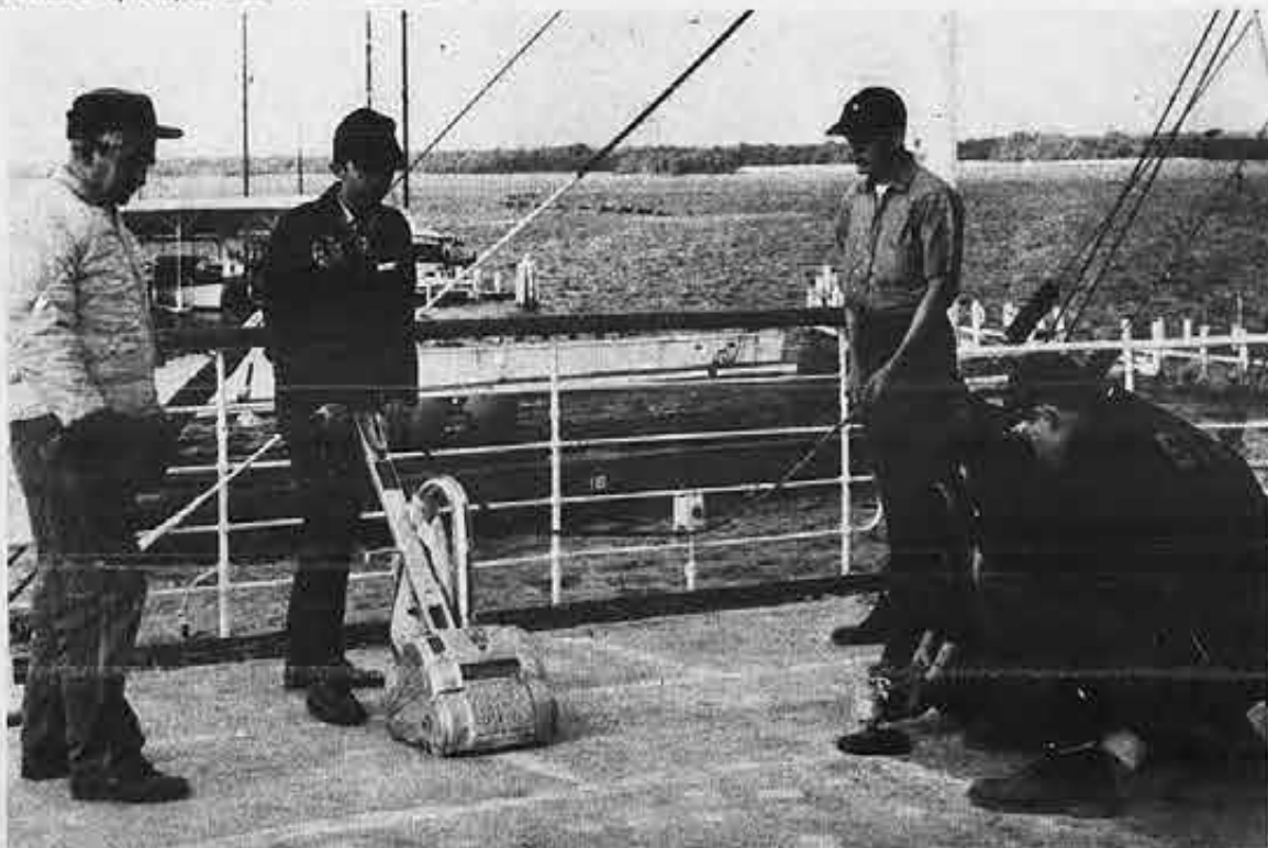
Deck trainees sand down seams on the newly-fiberglassed decks. All deck and engine work is supervised by experienced rated Seafarers.
