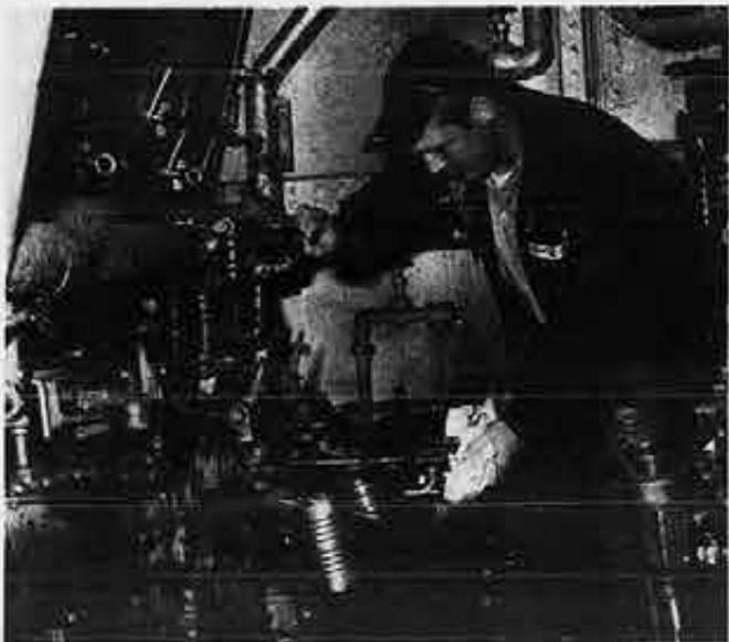
Trainee installs a burner in the ship's fire room. Trainees become thoroughly familiar with wiper's duties during their assignment aboard the Dauntless.
