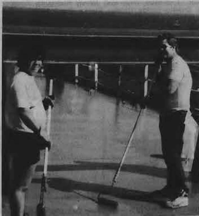
DEU Cilverio Wilson (left) and AB Mike Marquette help give the deck a new coat of paint.
