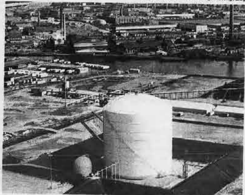
The LNG carried by these new ships will be stored in special tanks like this one in Brooklyn, N.Y., until needed during peak gas consumption periods, when it will be converted back to its gaseous state and piped to the consumer.
