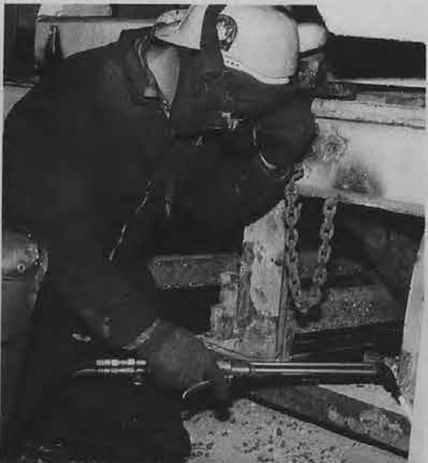
Conveyor belt roller replacement requires working in tight spaces as Conveyorman John Frankovich knows well.
