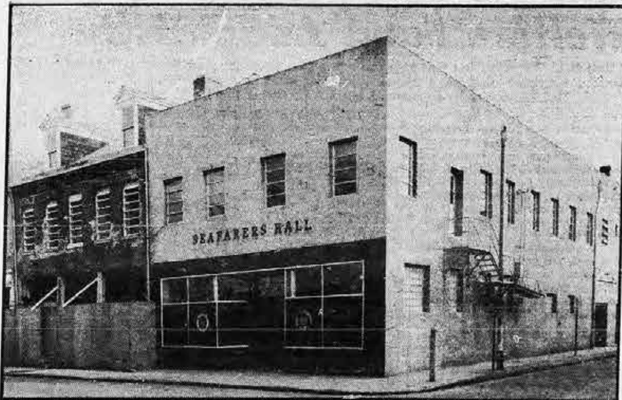
Work is underway at building (left) adjoining Mobile SIU hall. Added space will be used for Sea Chest retail and wholesale facilities, snack bar, TV room, and dormitory with laundry and shower facilities.
